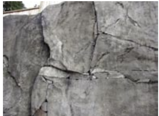
Fig. 8: Close-up of carved granite. SE 228th Street retaining wall, Sammish, WA, was the Washington Aggregate and Concrete Association Artistic Merit award winner
