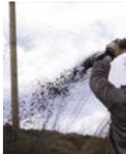
Example of poor velocity
