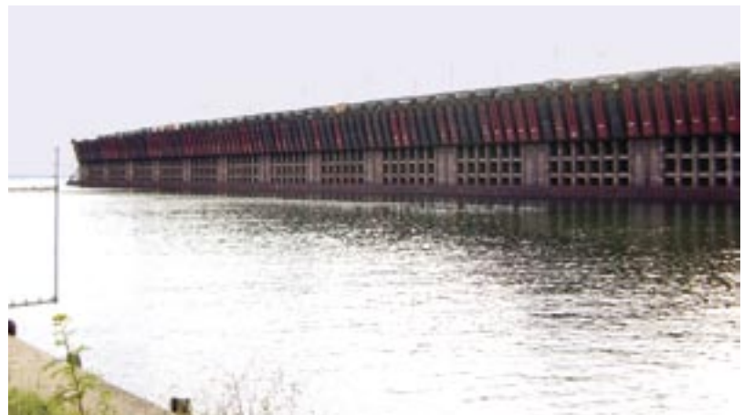
One side of dock showing sequence of columns needing extensive repairs
