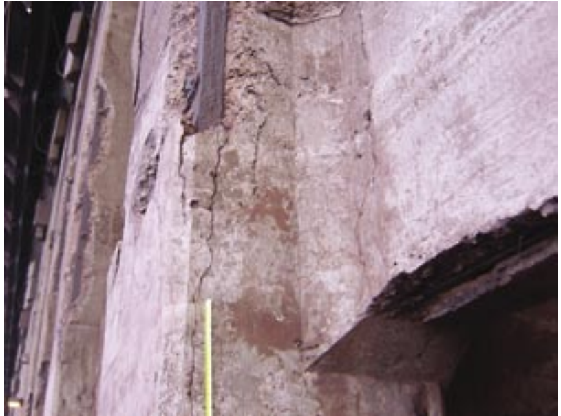
Close-up of damages to concrete support column and cracked concrete beam
