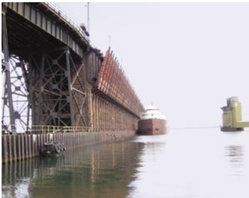
Overview of ore dock concrete support columns with barge taking on ore
