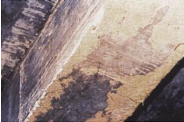
Underside of beam with sawdust before repair began
