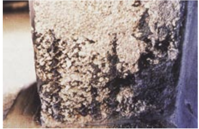
Honeycombed column-to-beam connection before repair
