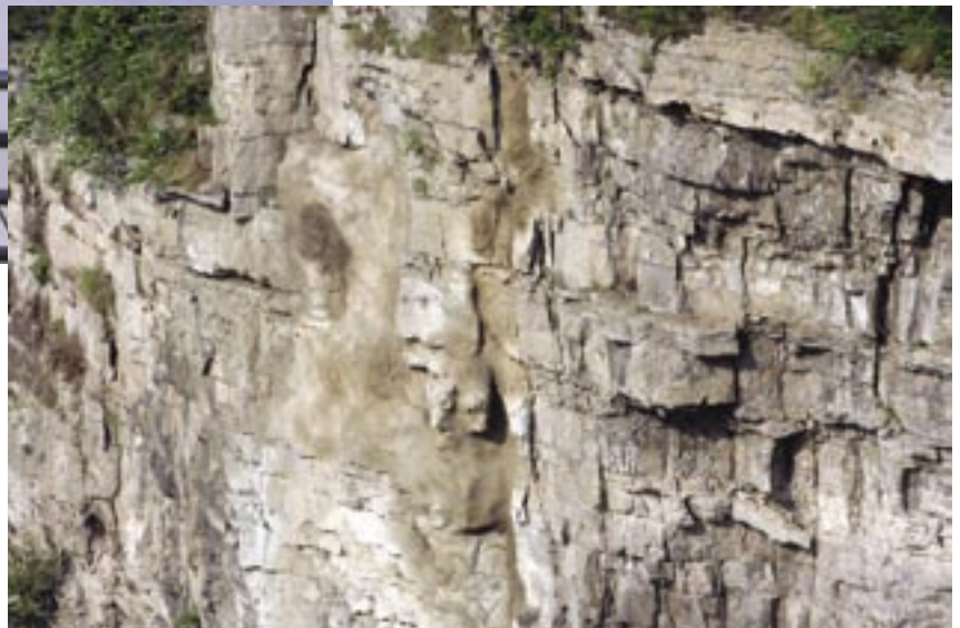
See how the loose column of rock is tied back into the slope using shotcrete
