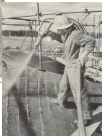
Fig. 3: Incorrect nozzling technique
