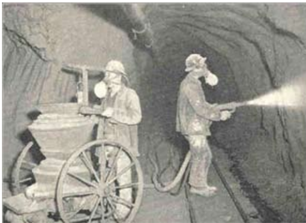
Fig. 1: Correct dry-shotcrete nozzling technique, 1916 (This photo is also found on the cover of Shotcrete, Winter 2003, V. 5, No. 1)
