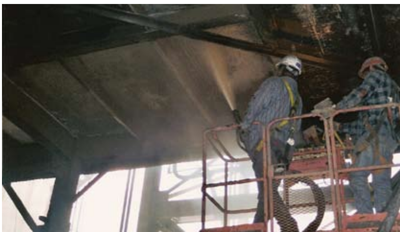
Overhead shooting on the underside of an elevated structure at the United States Steel, Clairton Works.
