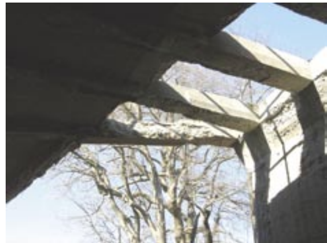
Typical deterioration of the supporting floor beams on the western side of the flyover
