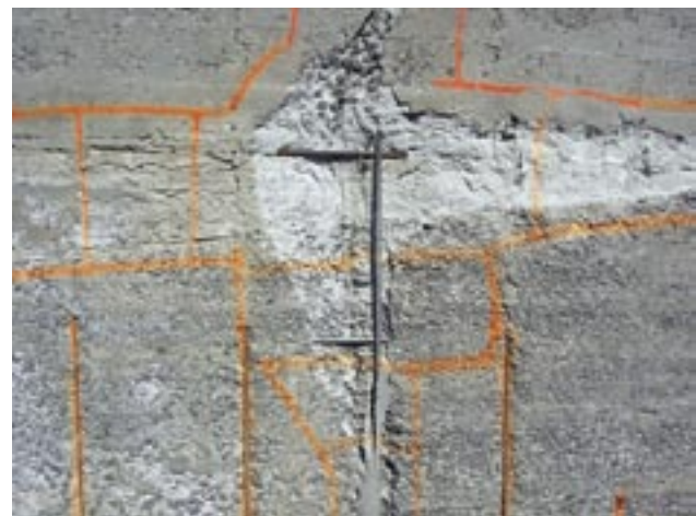
Typical cold joint with exposed reinforcing steel. Orange paint indicates limits of delaminations
