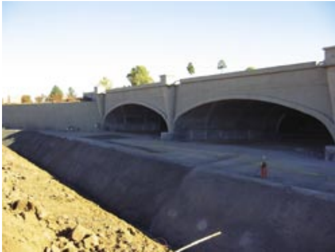
Shotcrete used in construction of headwalls, wing walls, arch, and cutoff wall
