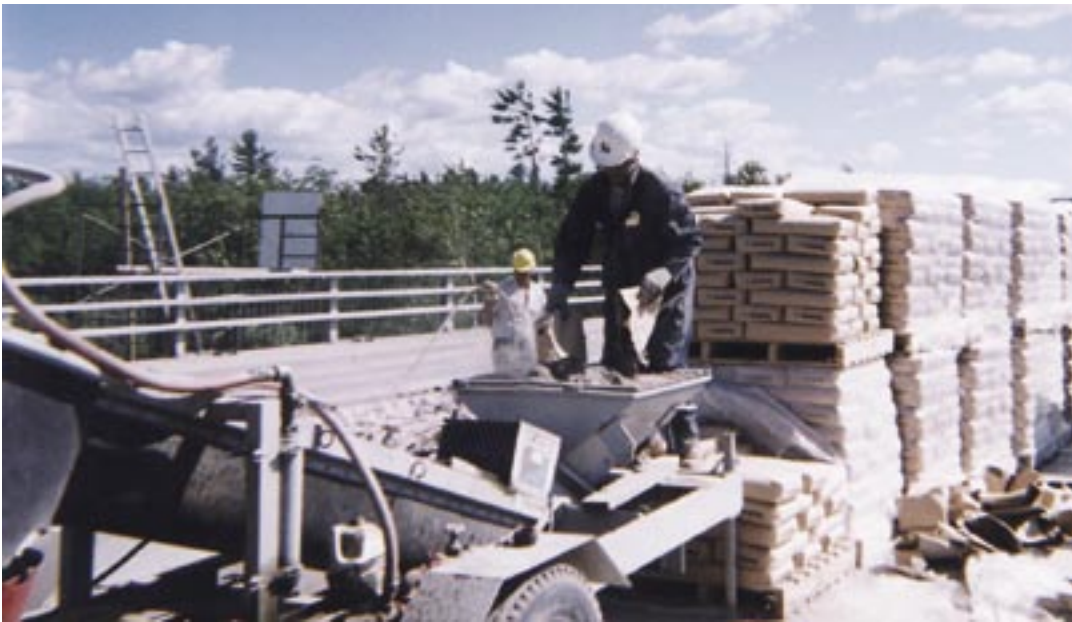
Fig. 2: Dry-mix prebagged shotcrete used with predampener for repairs to Hydro-Québec Dam in Fort Coulonges, QC
