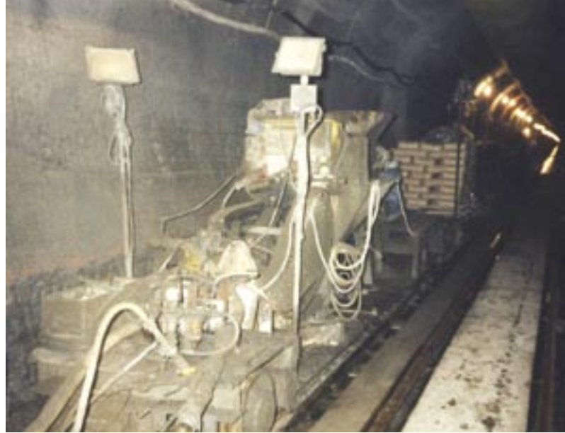
Fig. 6: Shotcrete equipment platform with air-operated pump, mixing auger, and prebagged shotcrete for Grondines Tunnel under St. Lawrence River; Lotbinière, QC
