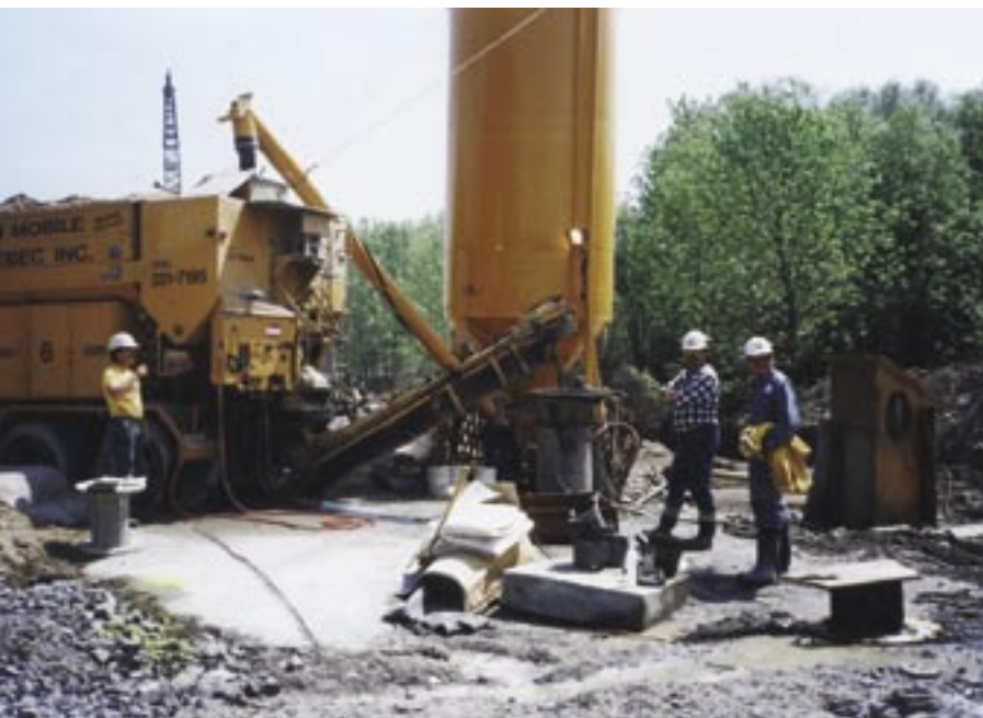
Fig. 4: Stationary concrete mobile mixer supplying wet-mix shotcrete for effluent outfall tunnel, Bécancour, QC
