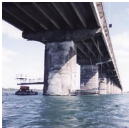
Fig. 1: Dry-mix prebagged shotcrete applied from marine installation for pier repairs on Champlain Bridge, Montréal, QC
