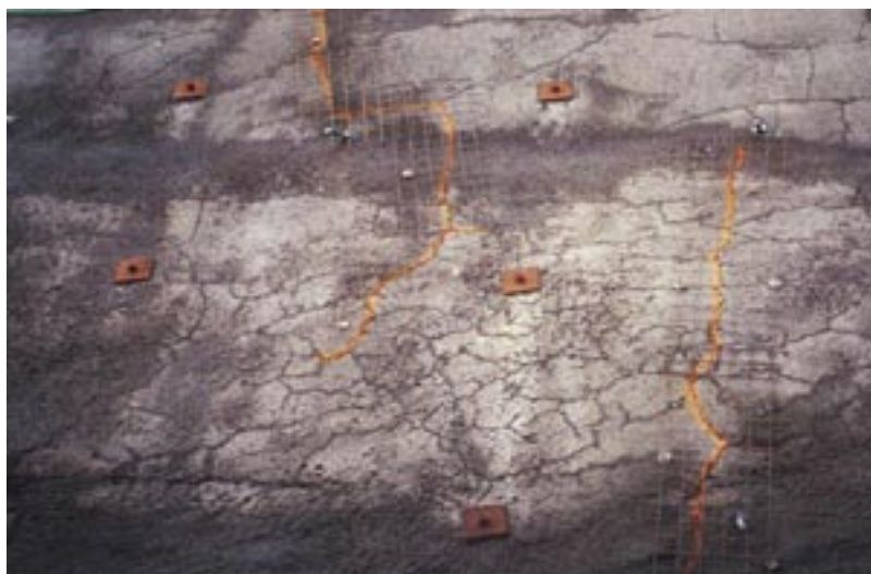
Cracking as a result of shotcrete not properly cured
