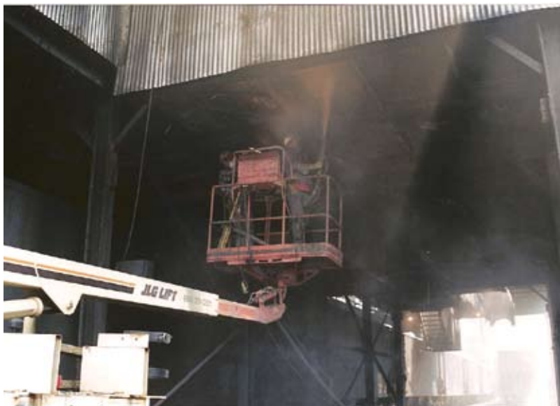
Overhead shooting on the underside of an elevated structure at the United States Steel, Clairton Works, Clairton, PA
