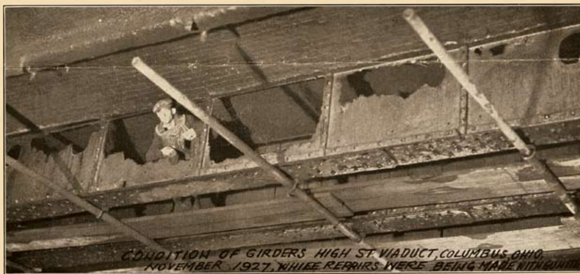
Fig. 1. Condition of girders, High St. Viaduct, Columbus Ohio, November, 1927, while repairs were being made with "Gunite"
