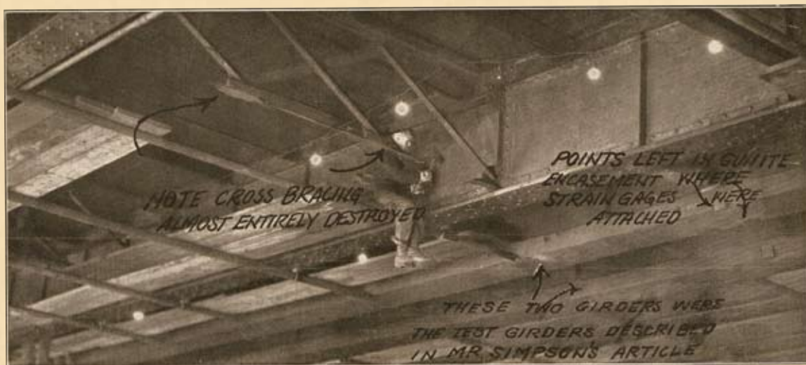
Fig. 2. Shows test girders described in Mr. Simpson's Article. Also note Cross Bracing almost entirely destroyed.
