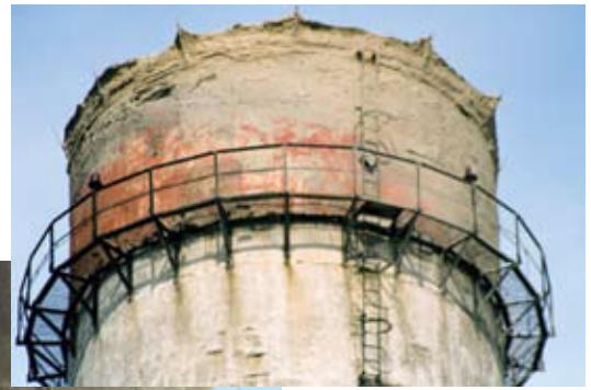
Damaged chimney capital before repair
