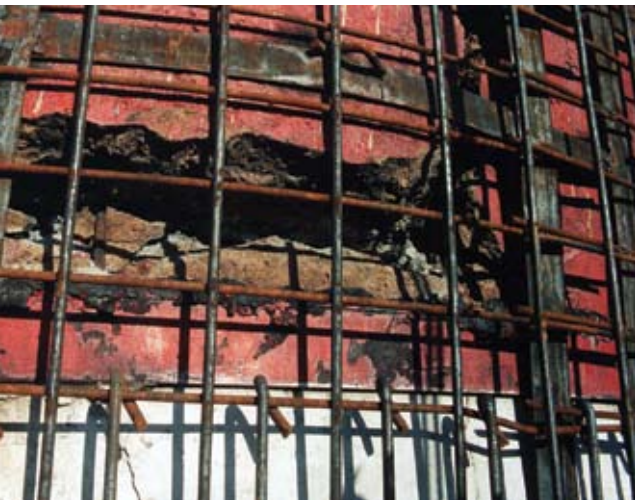
Damage of chimney shaft (500 ft [150 m]) high at the height of approximately 425 ft (130 m)
