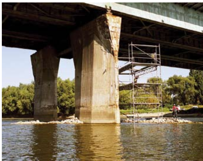
Corrosion damage of bridge support
