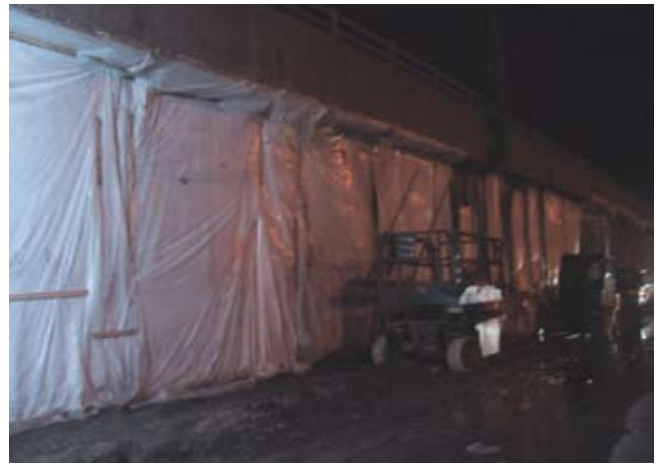
Fig. 10: Synthetic fiber burlap, saturated with water, covered with a polyethylene plastic sheet
