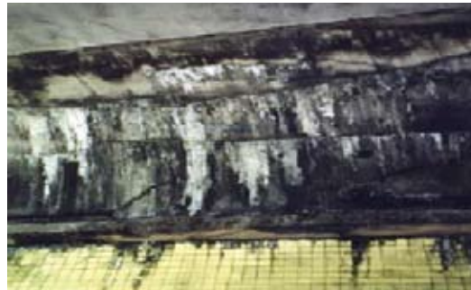
Station 14+50—horizontal cracking of arch
