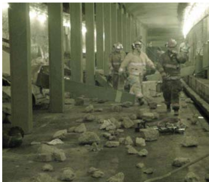
Collapsed tunnel training area
