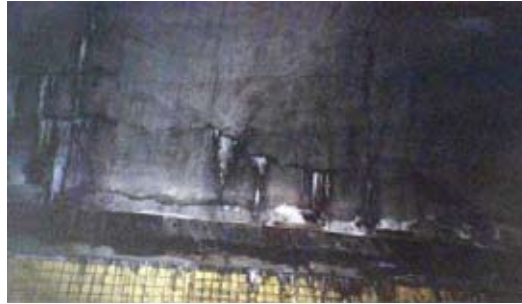
Typical leaking crack in tunnel arch
