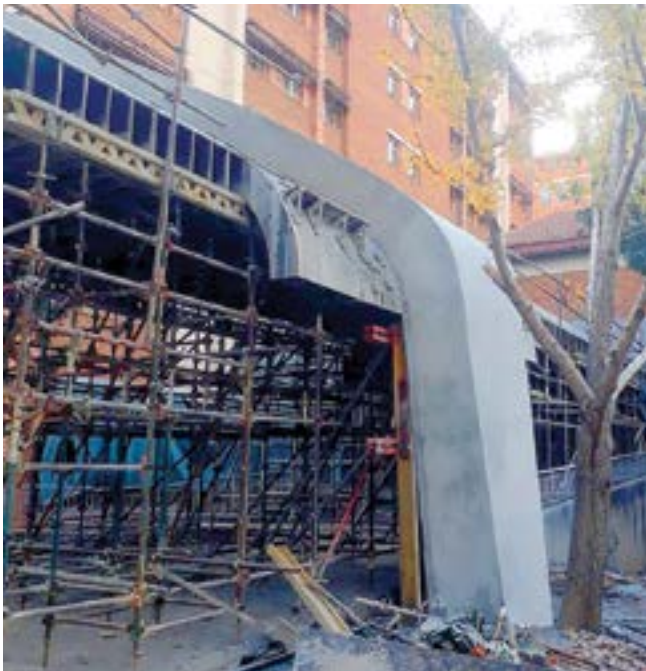
Fig. 5: A view of the curved column with canopy sitting on the form
