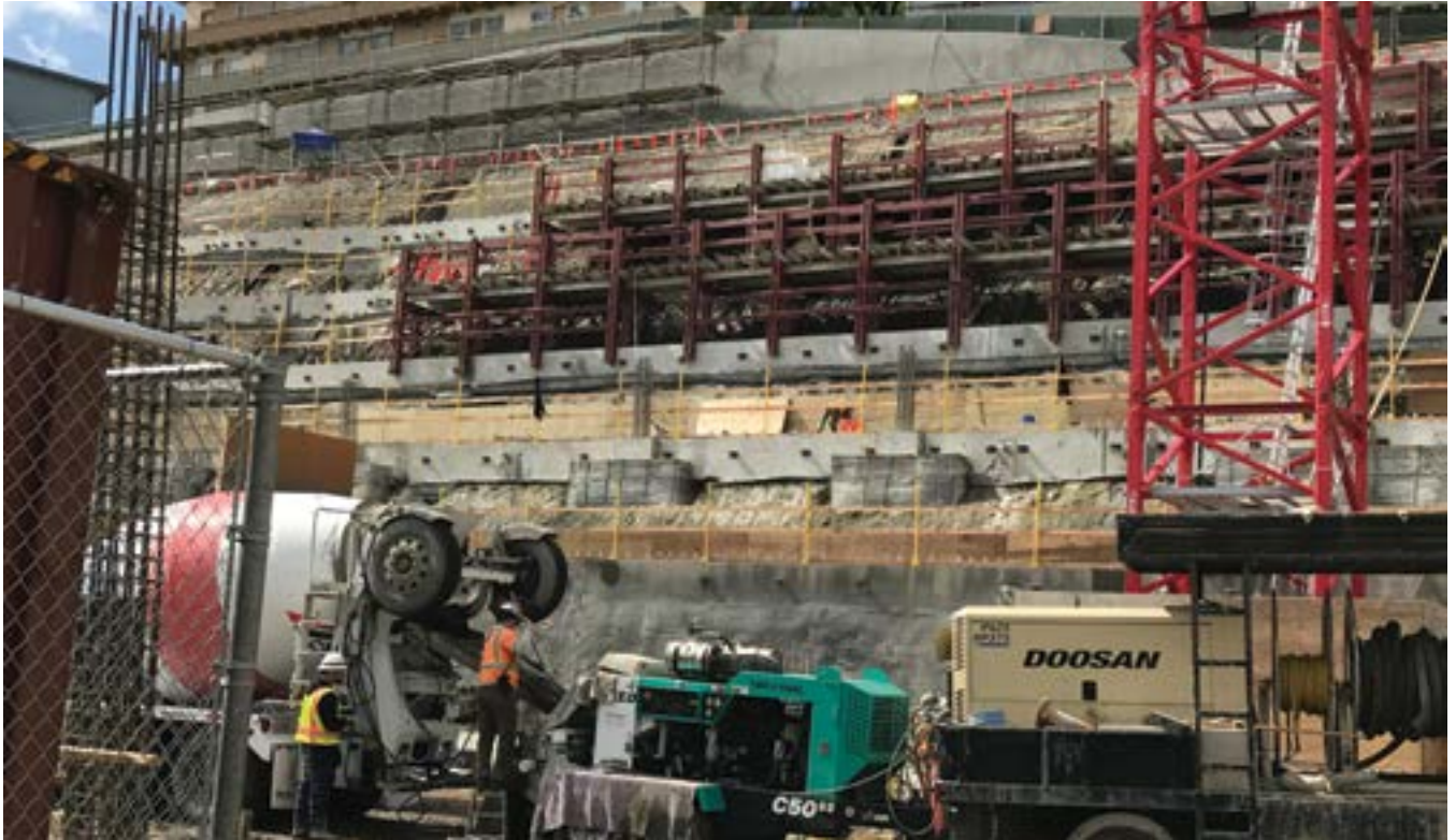
Fig. 5: View of the jobsite with multi levels of grades beams and rear retaining wall to the project
