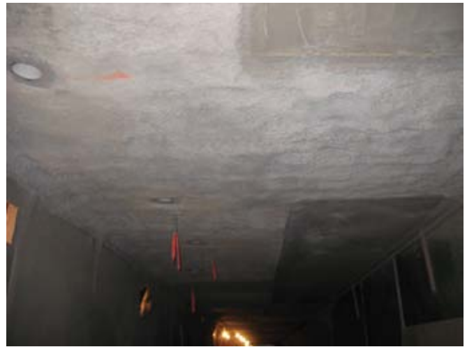
Core testing for bond and compressive strength was taken from these locations
