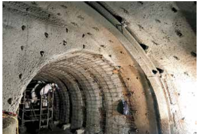
Fig. 5: First layer of shotcrete installed with preexisting support bents still in place
