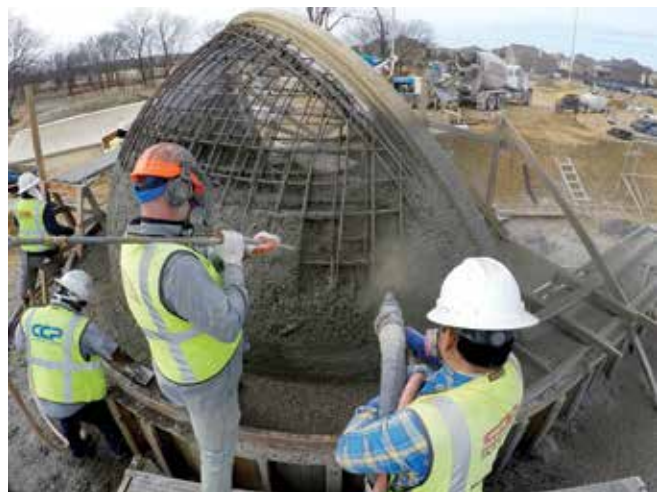
Fig. 6: ACI Certified Nozzleman and blow pipe operator. Stucco lathe placed between reinforcement curtains. Shotcrete pump and equipment in background
