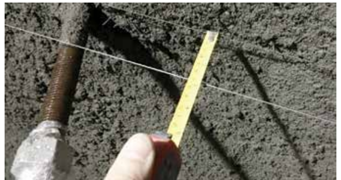
Fig. 20: A 1 in. diameter anchor embedded in shotcrete and shooting wire positioned to show nozzle thickness to build out next layer of shotcrete
