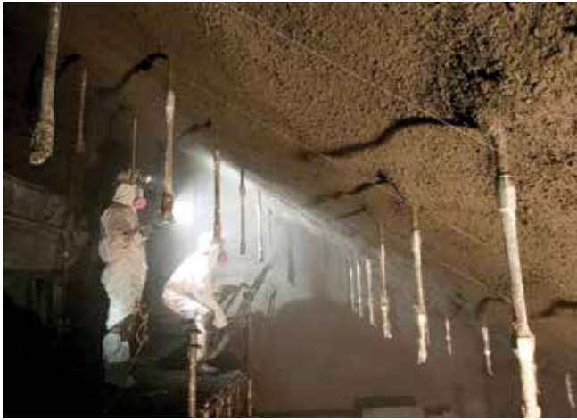
Fig. 17: Nozzlemans shooting overhead on scaffold platform in crouching position maintaining adequate shooting angle and distance to receiving surface and building out shotcrete to shooting wires
