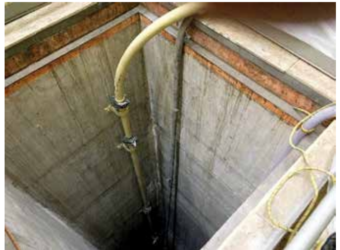
Fig. 15: Steel line entering draft tube from powerhouse
