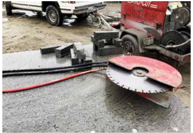
Fig. 10: Diamond wire-cut section of full-scale mockup showing excellent shotcrete consolidation around reinforcing bar and saw-cut prisms for bond testing
