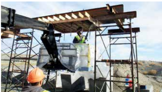
Fig. 7: Nozzleman building out shotcrete to cover reinforcing bar and around anchor rods of preconstruction mockup
