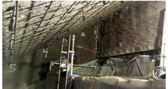
Fig. 19: Concrete substrate, formwork, 1 in. anchors, and No. 5 reinforcing bars installed and ready for shotcrete application
