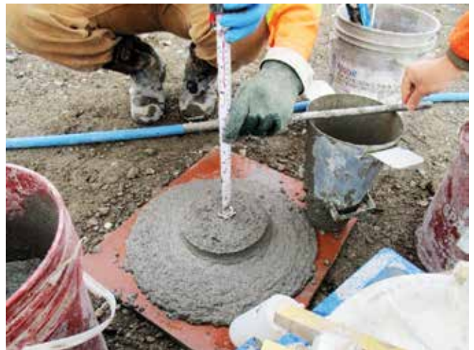
Fig. 11: Slump of approximately 9 in. confirmed based on testing in accordance with ASTM C143/C143M
