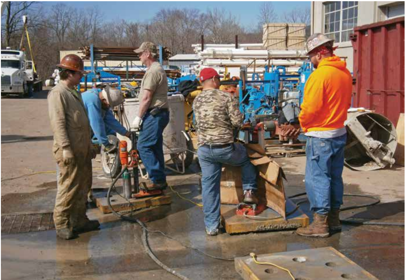
More than one core drilling rig with crews who have experience in the operation
