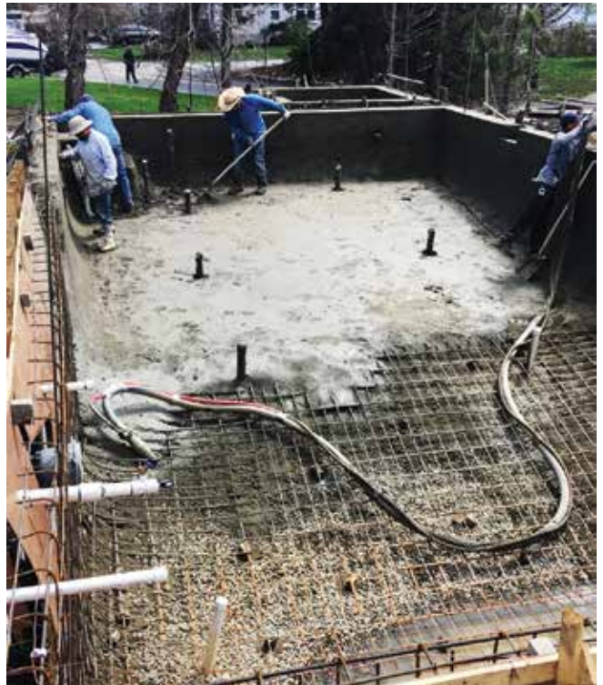
Fig. 2: The crew is able to walk on recently shot dry-mix material without sinking into the surface
