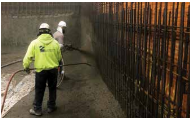
Fig. 4: The same pool shown in Fig. 3 contained over 55 tons (50 tonnes) of reinforcing bars. With an extremely tight schedule, wet-mix easily allowed placement of concrete in 5 days
