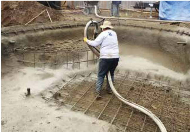
Fig. 5: SSG used dry-mix shotcrete for this smaller pool with about 50 yd 3 (38 m 3 ) of concrete and easily completed in 1 day with dry mix. Additionally, the steel schedule was light and with a tight jobsite it is easier to clean up a dry-mix setup than a wet-mix setup
