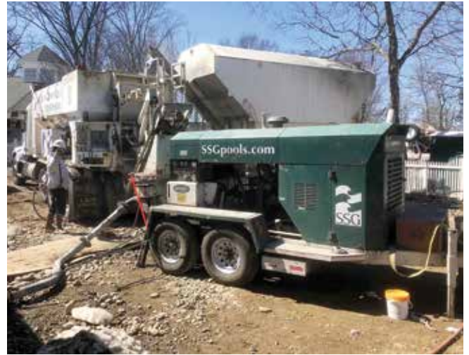
Fig. 6: Wet-mix shotcrete pump and on-site volumetric mixer allowed for faster production, as there was no swapping out of concrete trucks
