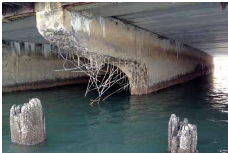
Fig. 2: An example of a severe girder repair
