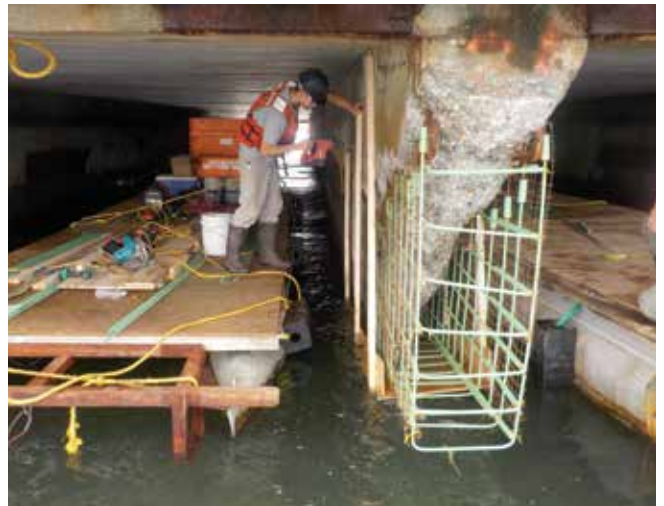
Fig. 4: The installation of a wooden form to help create the right taper of the girder bottom
