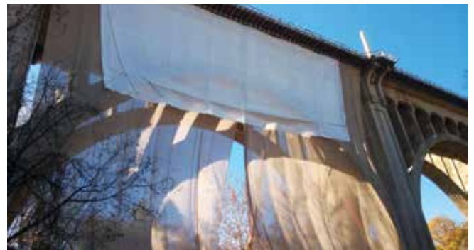
Fig. 8: Burlap and reinforced poly curtains sewn together and hung from cables to protect cars and buildings from overspray
