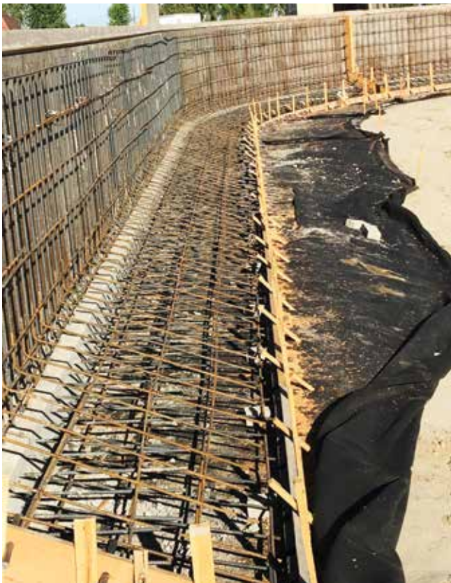
Fig. 1: Reinforcing bar and formwork prior to shooting condition at south wall, where wall and slope were shot monolithically
