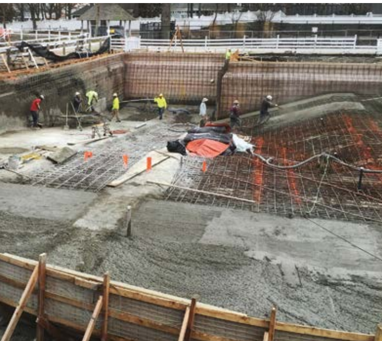
Fig. 3: Shotcrete installation—4 ft (1.2 m) wide strips being installed and the 10 ft (3 m) wide openings to be filled in later
