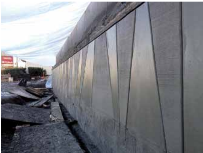
Fig. 4: Retaining wall with an architectural pattern of radiating reveals, with alternating broom-and-polished finish
