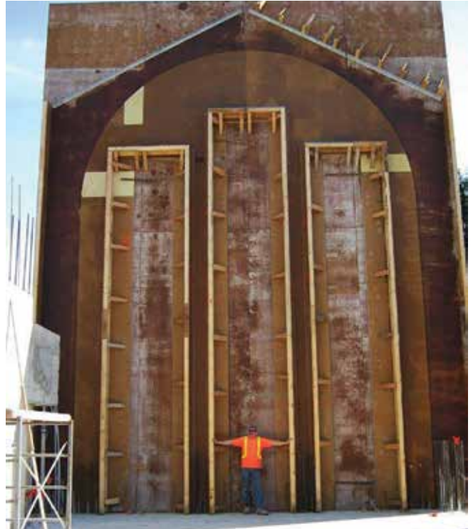
Fig. 5: Complex shoot panel formwork for a church; notice the lack of internal bracing required in the window breakout
