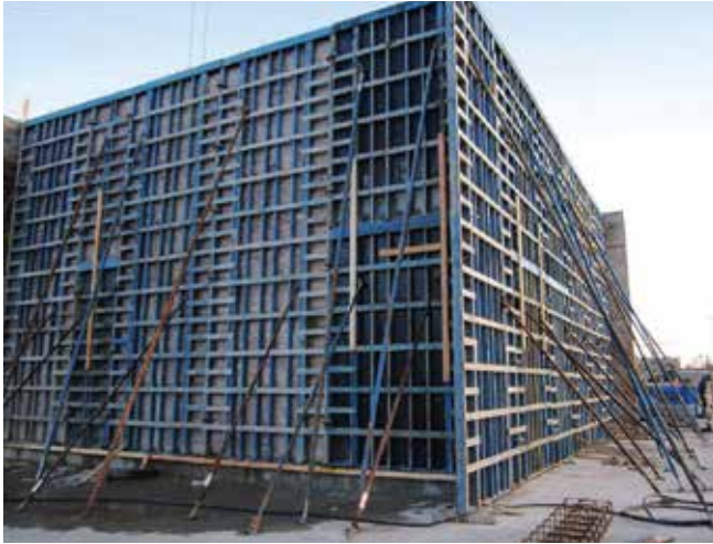
Fig. 7: Tall, light one-sided shoot panels with pinwheeled corners and uneven base; not possible with form and pour
