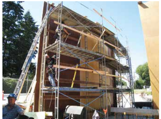
Fig. 2: Architectural reveals and recessed panels on single reskinned shoot panels for curved wall prior to reinforcing bar placement
