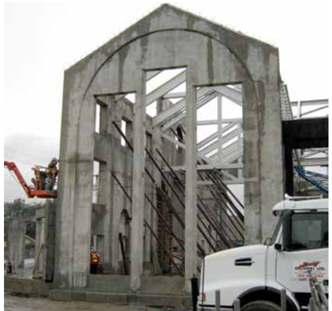
Fig. 6: Finished shotcrete structure using only one-sided shoot panels, eliminating the risk of voids in the slender pillars that can occur when using form-and-pour
