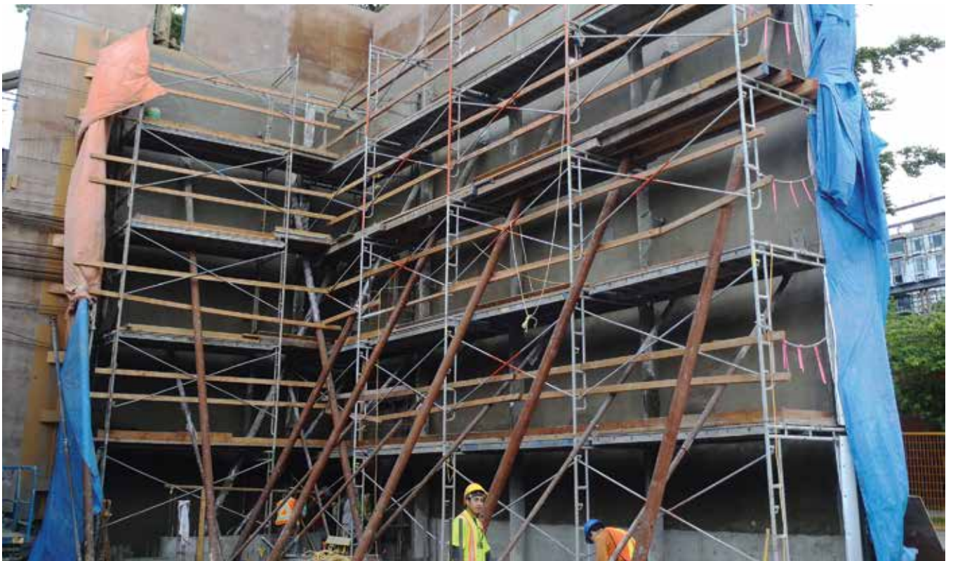
Fig. 8: Tall shoot panels braced from the shot side due to property line constrictions
