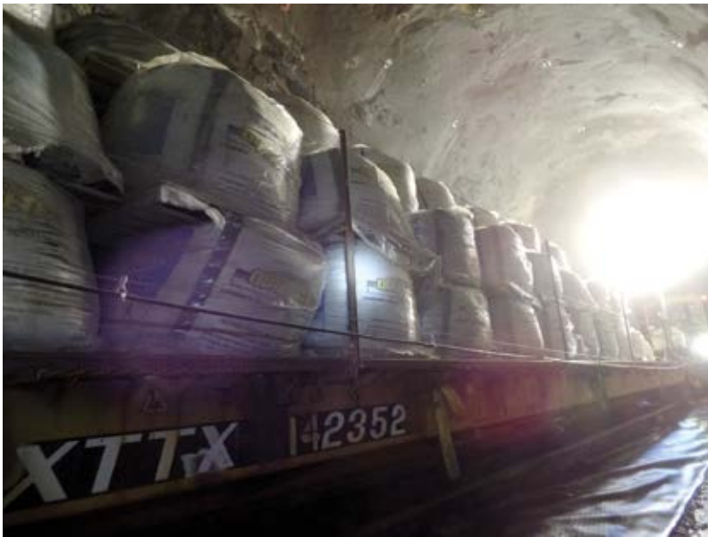
Fig. 5: Fifty bulk bags loaded on a flat car for final liner installation
