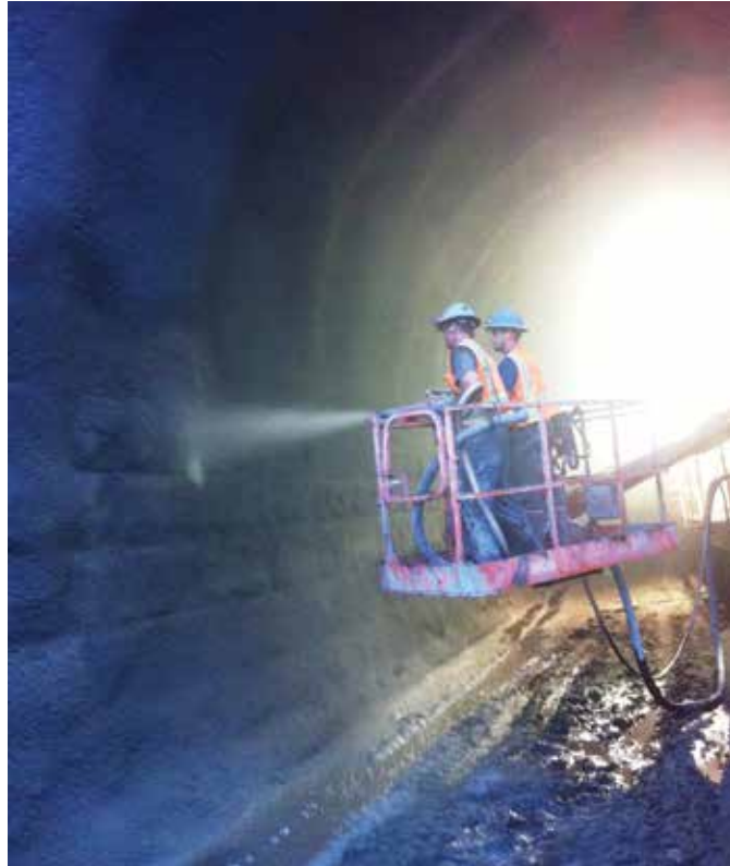
Fig. 3: Manlifts used to access the arch roof for scaling, drainage placement, and shotcreting
