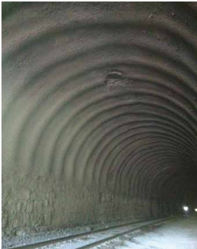
Fig. 1: Ribs 8 in. (203 mm) thick with 4 in. (102 mm) of shotcrete in between were placed
