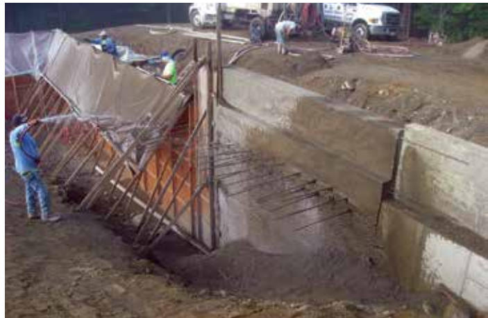
Fig. 3: Deep excavation required for forming and, subsequently, filling with free-draining stone to prevent frost heave. Also seen is the dowel reinforcing bar that was tied into the pool floor in the second phase
