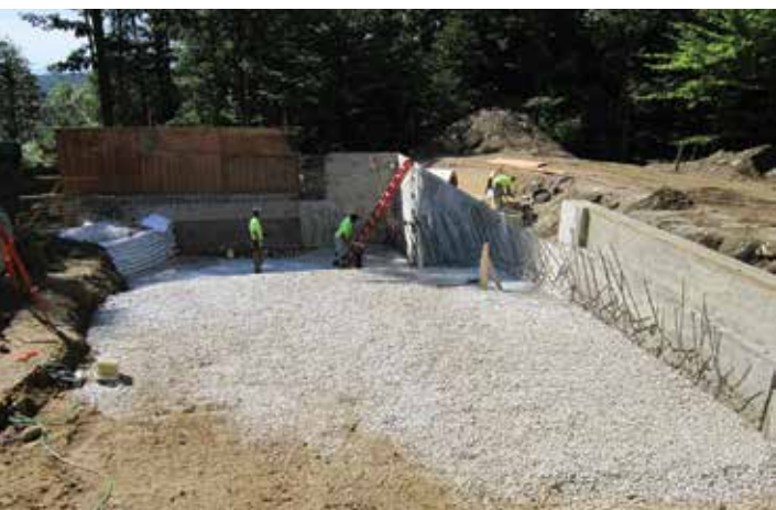
Fig. 1: Stone underlayment along with the reinforcing bars penetrating out of the first phase of construction so the second-phase pool section could be tied in correctly
