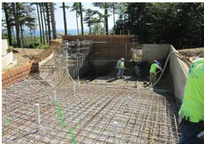
Fig. 2: Elaborate reinforcing required by the pool design as we start the second phase of shotcrete
