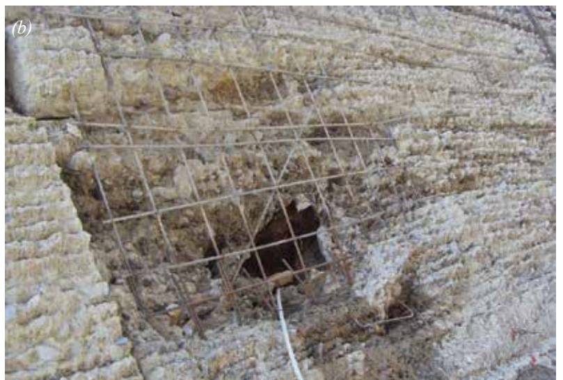
Fig. 2: Challenge of hydrodemolition at a multi-curved spillway: (a) robotic head at a curved surface; and (b) after hydrodemolition
