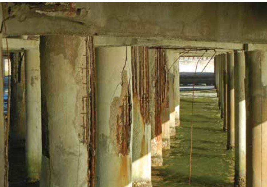
Fig. 1: Deteriorated columns between water line and deck
