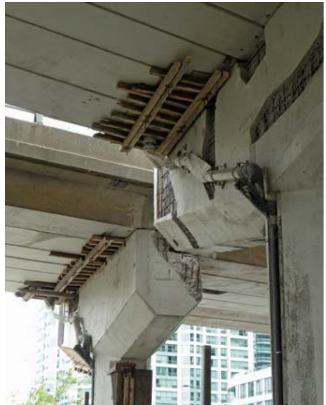
Fig. 3: On elevated structures, forms and form hardware must be lifted into place and removed several days later
