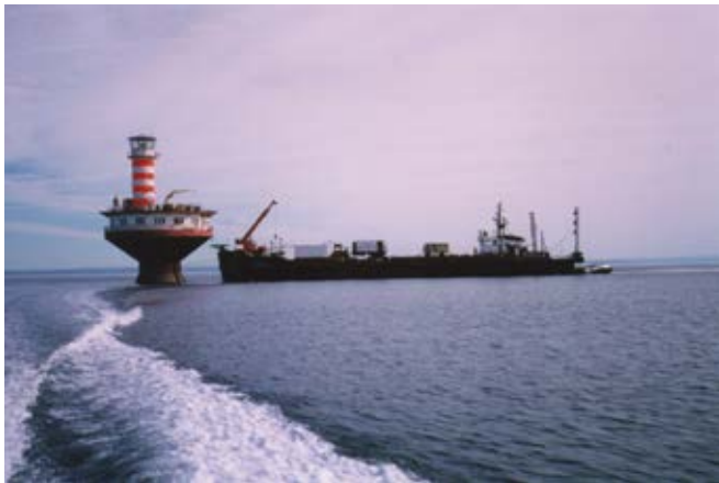
Fig. 4: Shotcrete was specified as the concrete placement method for the rehabilitation of the Haut-fond Prince Lighthouse in the St. Lawrence River
