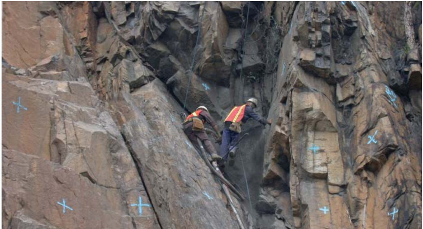
Fig. 6: In addition to being skilled in the art of dry-mix shotcrete placement, the AUSL nozzlemen had also mastered the skill of rappelling down rock faces
