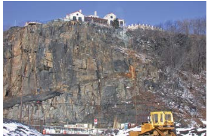
Fig. 5: New Jersey Transit was faced with the challenge of stabilizing the rock face of the King's Bluff Slope
