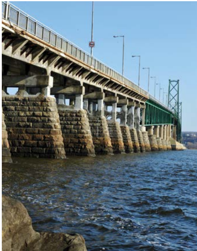
Fig. 2: The rehabilitation of elevated bridge structures is a common example of an application where the shotcrete process can minimize the problems related to access
