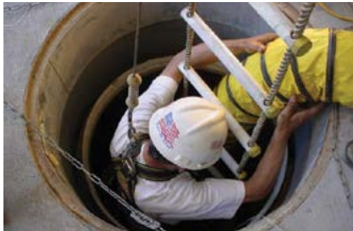
Fig. 1: Worker entering a manhole opening into a confined space along the side of a ventilation tube
