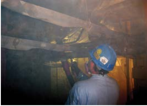
Fig. 4: Nozzleman shooting overhead in a tightly confined area. In areas where visibility and ventilation are concerns, adequate lighting should be provided and the appropriate personal protective equipment should be worn
