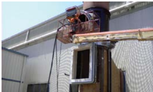
Fig. 2: In confined areas like this steel mill smokestack and ductwork, a refractory lining is being gunned in place using the dry process
