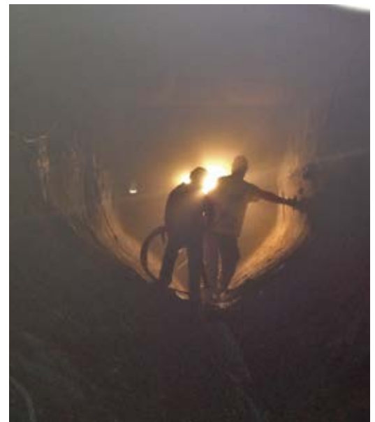
Fig. 3: In this confined space area in a power plant ash pit, dry-process shotcrete is being gunned in place
