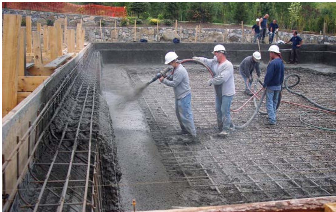
Proper shotcrete placement requires everyone, from the pump operator to the nozzleman, to know his role
