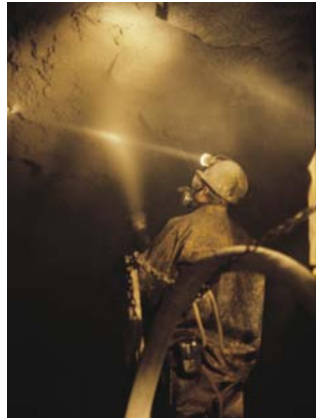
Nozzleman applying shotcrete to back in order to provide ground support during the mining process
