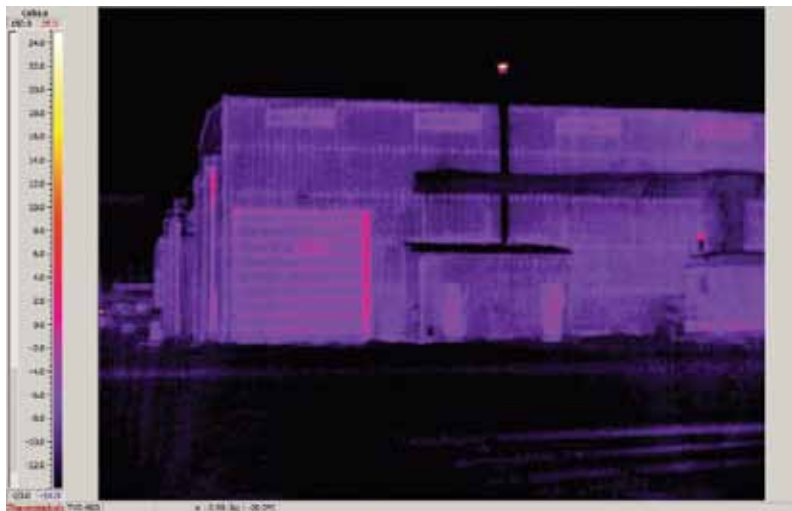
Fig. 5: Thermographic photo of steel building showing significant heat loss
