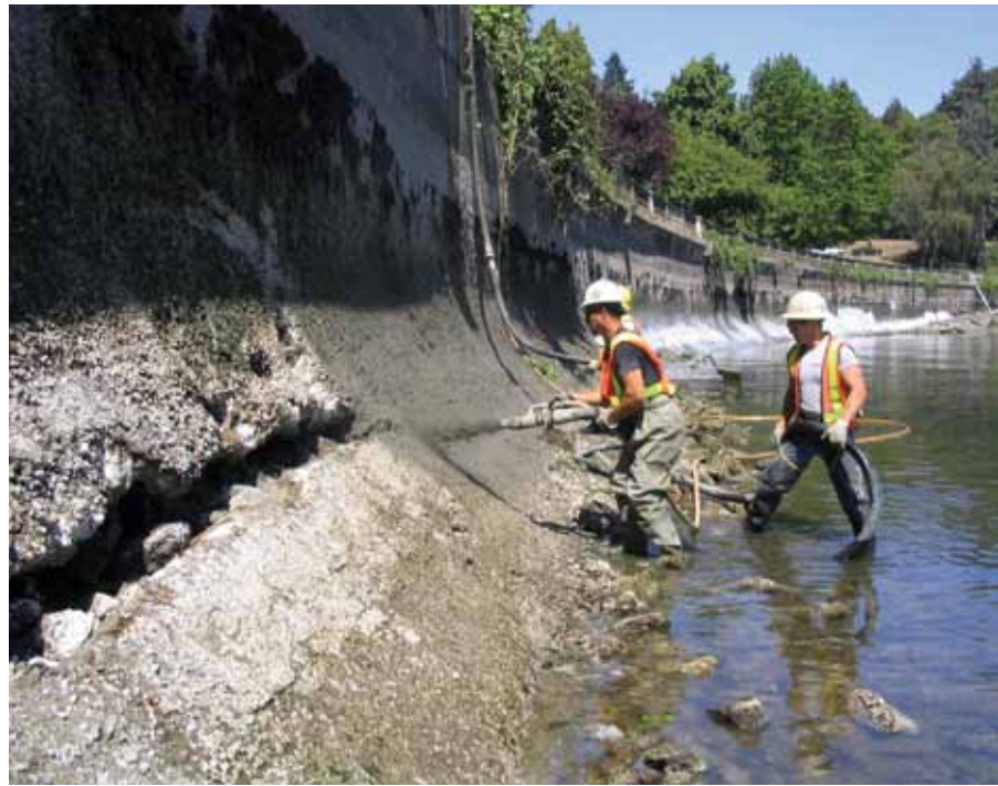
Fig. 5: Shotcrete repairs to damaged concrete faces rip-rap in the Devonian Park part of the Stanley Park Seawall in Vancouver, BC, Canada Photo courtesy of D.R. Morgan
