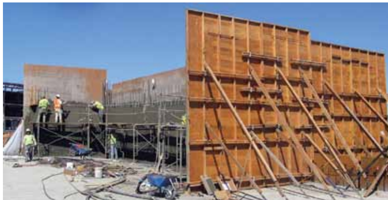
Fig. 1: Single-sided plywood formwork set up as a shotcrete receiving surface in California
