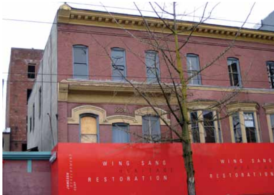
Fig. 6: Seismic retrofit of the 100-year-old Wing Sang Building in Vancouver, BC, Canada
