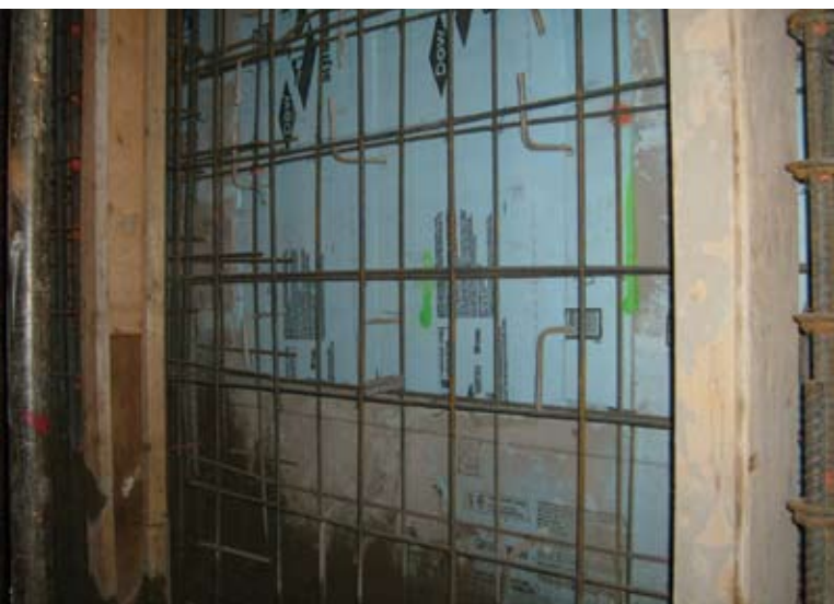
Fig. 8: View of a typical wall section with L-bar dowels, reinforcing bars, and pilaster edge forms installed
