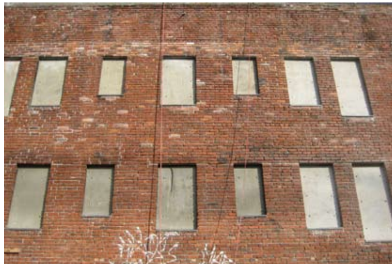
Fig. 4: View of upper level of north building, note windows filled with reinforced shotcrete
