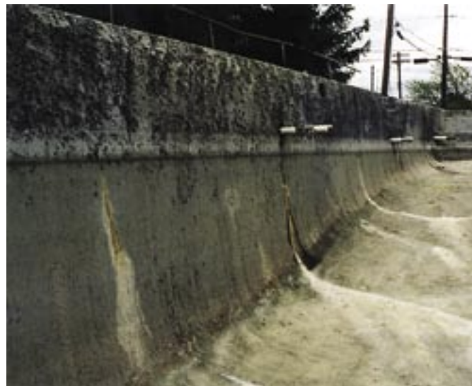
Fig. 4: Cracks observed in main pool of New York apartment complex
