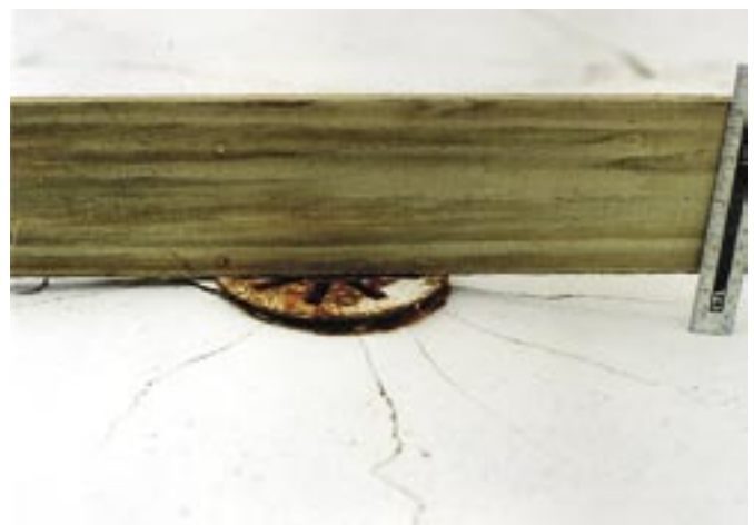
Fig. 6: Measuring movement of water inlet above floor level
