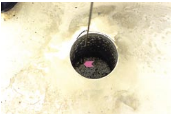
Fig. 5: Wire probe inserted into the space between the original substrate concrete and shotcrete shell
