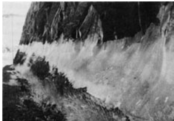
Conventional shotcrete placed adjacent to a major highway. The environmental consideration may be questioned
