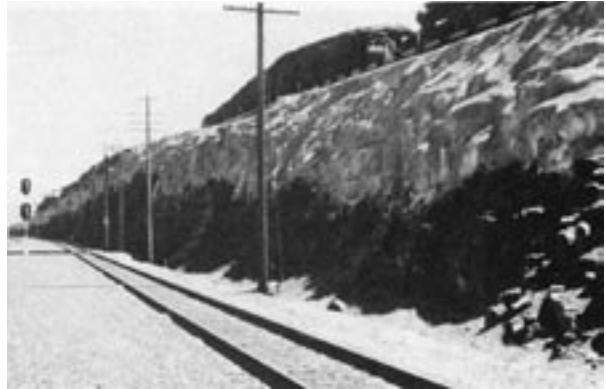
Conventional shotcrete placed adjacent to a major railroad. Aesthetics may have been improved if colored shotcrete would have been used
