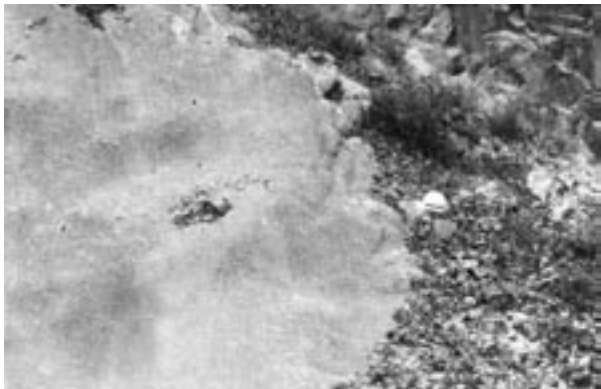
Colored shotcrete adjacent to a project access road, Lower Granite Lock and Dam
