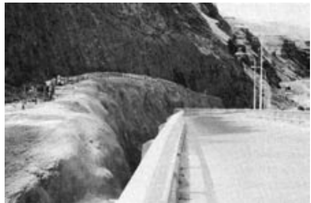
Colored shotcrete adjacent to a roadway at Lower Granite Lock and Dam, Snake River, Washington. Shotcrete placed as rock slope stabilization
