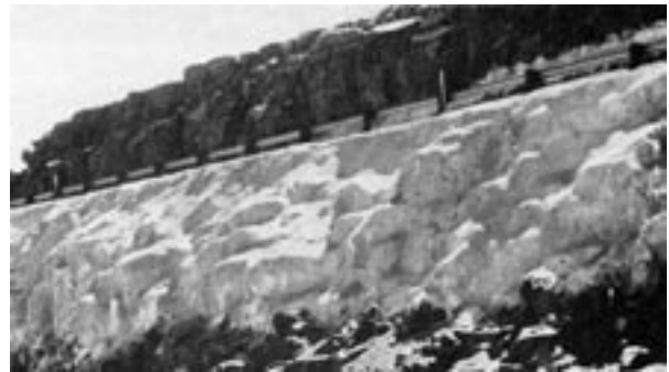
Conventional shotcrete placed below a major highway but adjacent to a major waterway
