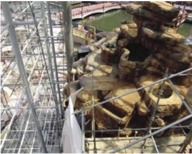
Shotcrete rockwork is directly adjacent to delicate exterior glass walls. Massive pockets in the rock formations will accommodate plants and trees
