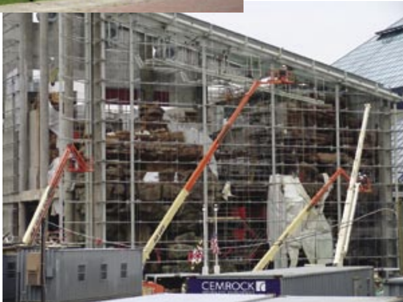
The National Aquarium in Baltimore's recent expansion included creating monumental shotcrete mountains inside a contemporary glass building
