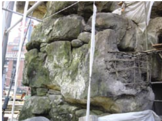
Shotcrete is applied over hand-bent reinforcing bar shapes then "carved" and painted to resemble the desired geology
