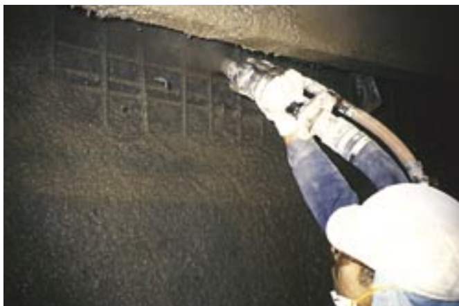
Fig. 6: Final closure of massive placements stopped short of overhead with beveled face, to allow shrinkage prior to final closure
