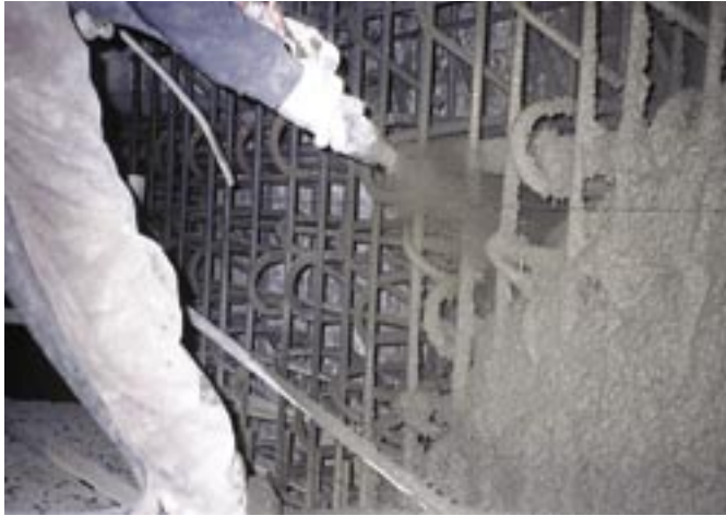
Fig. 8: Wet-mix process allows the nozzle to be held very close and even within the outer reinforcing to achieve complete encapsulation
