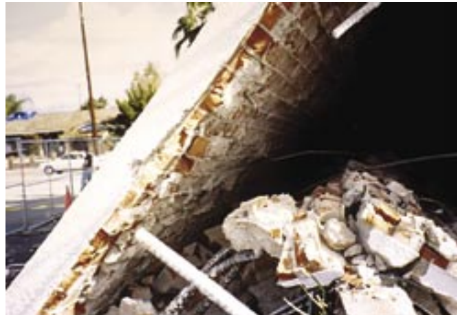
Fig. 10: The brick wall shattered but outer layer remained bonded to the shotcrete
