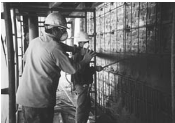
Fig. 1: Minimal reinforcing and fairly thin shotcrete augmentations were common in early seismic retrofit
