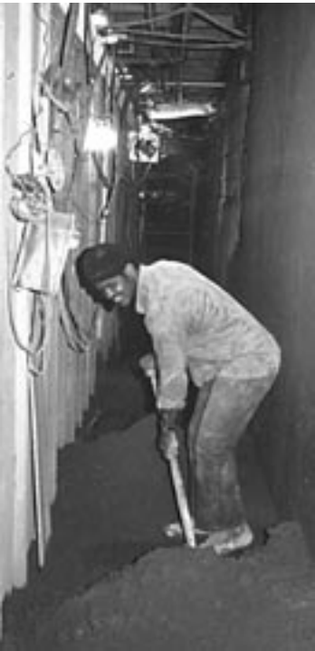
Fig. 5: Large amounts of rebound were produced, especially in cramped conditions with heavy reinforcing
