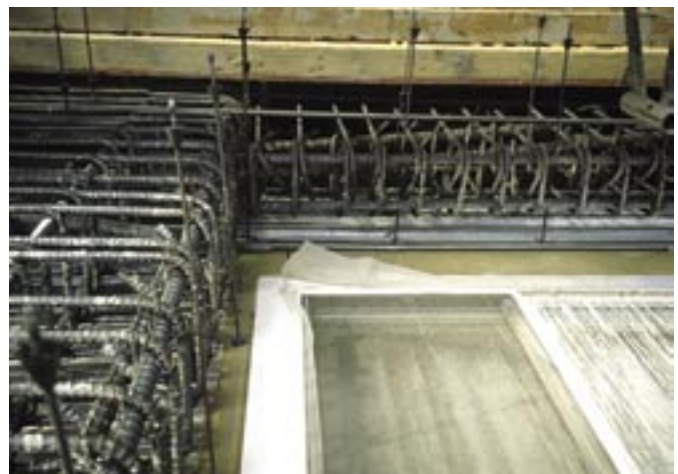
Fig. 7: The reinforcing for seismic retrofit continues to get larger and more congested
