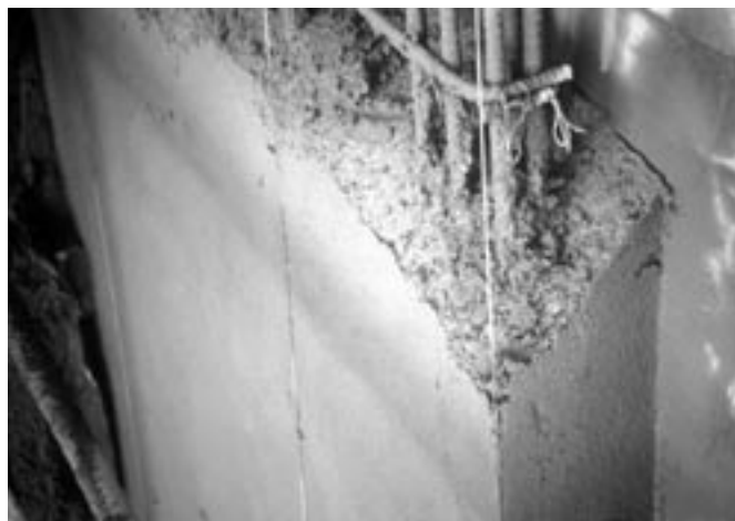
Fig. 2: Ground wires rather than forms were and continue to be used for maximum nozzle access
