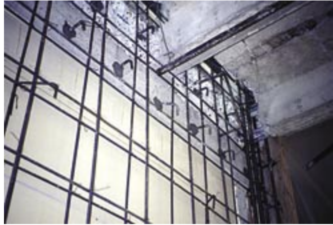
Fig. 3: Multiple reinforcing curtains and continuity between floors became common following the 1952 Tehachapi earthquake
