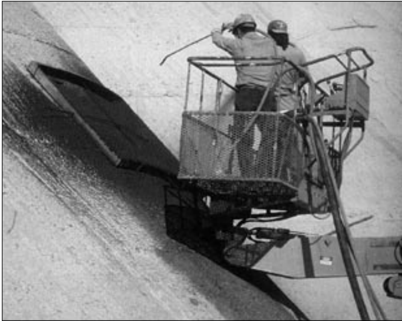
Fig. 3: General view of shotcrete application from a boom lift to test panel
