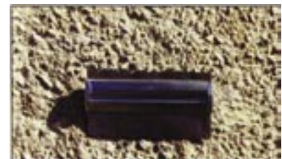
Fig. 1: Sandblasted concrete in the arch barrels. The profile gauge was used for measuring the surface roughness profile. Note the exposed texture of the prepared surface
