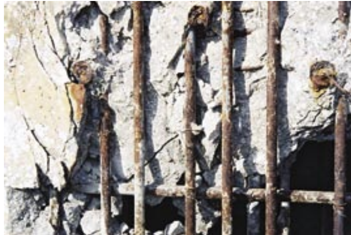
Fig. 3: Highly fractured concrete in the early stages of preparation
