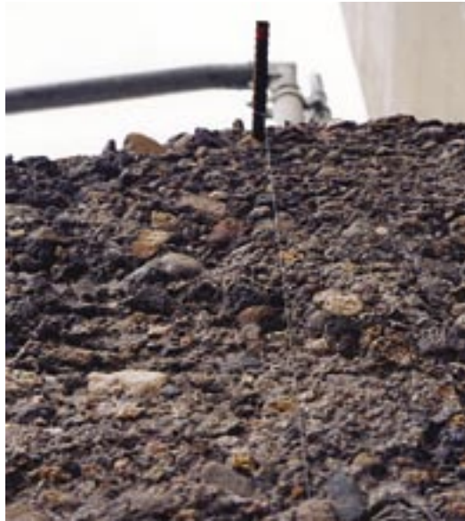
Surface prep via hydrodemolition method. Shoot wires stretched across area before wet-mix process shotcrete application
