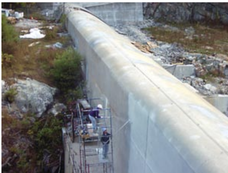
Fig. 1: On the upstream side of Blackwater Dam, cementitious waterproof coating is spray-applied and backrolled with two-coat application by Aulson crewmen
