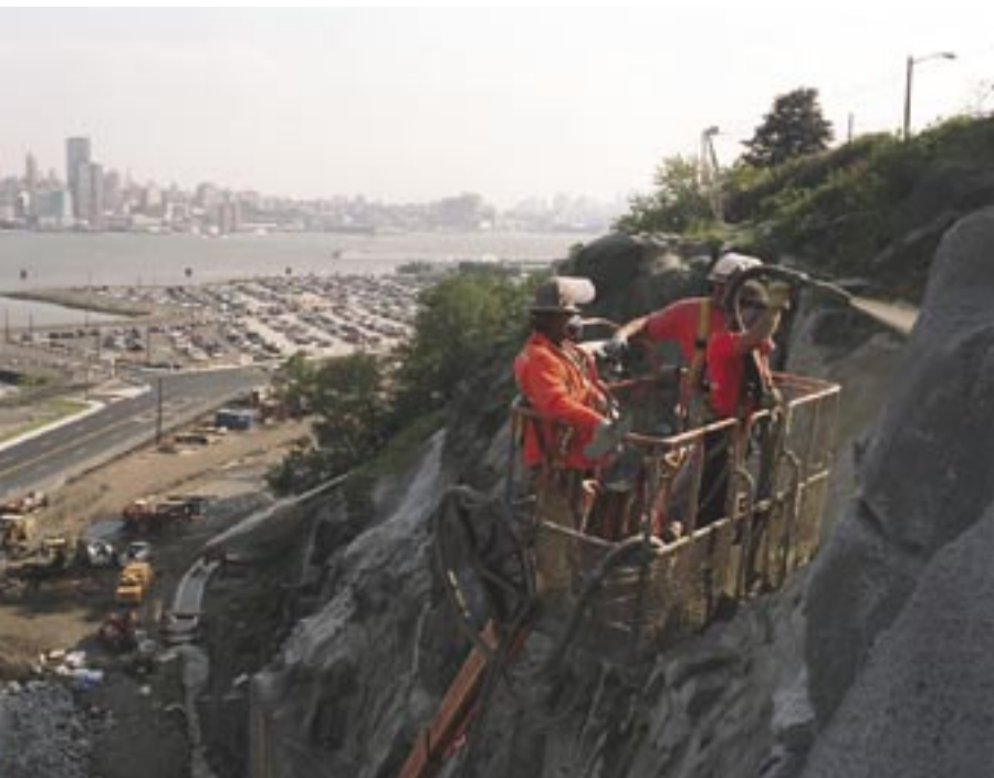
Application of wet shotcrete in preparation for sculpting at East Portal's gorilla's head landmark
